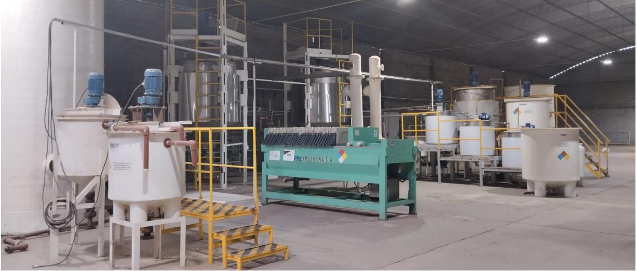
Figure 4: 250tpa Lithium Carbonate Pilot Plant in Salta, Argentina
