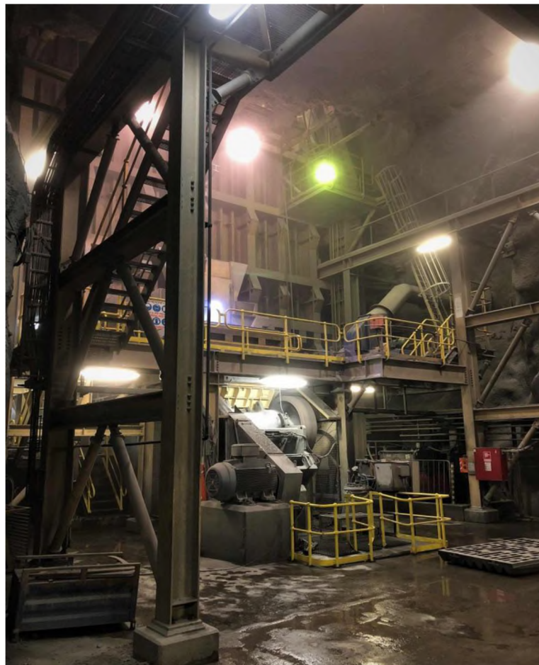
FIGURE 16-2: UNDERGROUND JAW CRUSHER STATION BENEATH THE ROM BIN, 165 LEVEL
