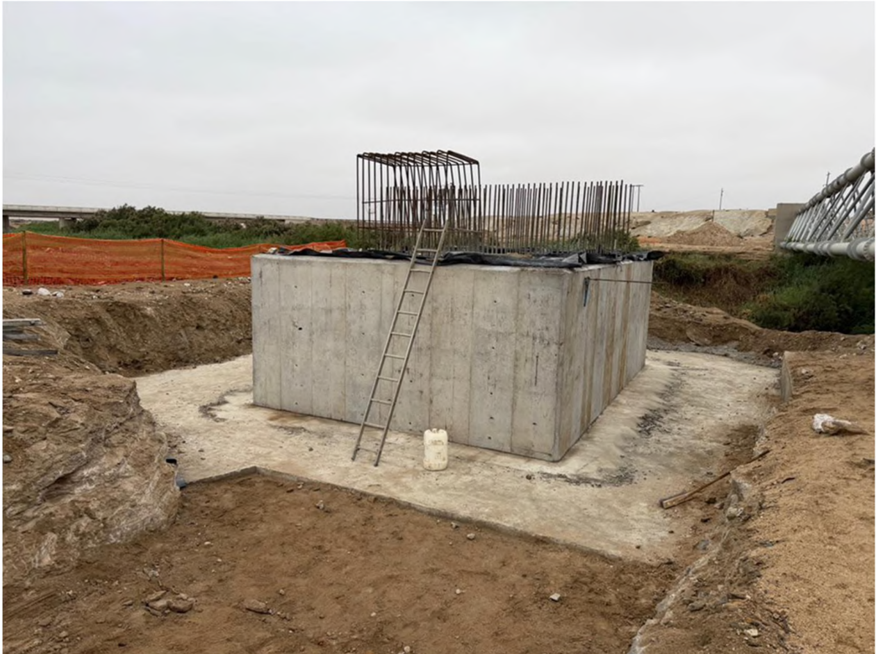
Figure 4: The permanent water supply pipeline bridge base to cross the Swakop River is nearing completion
