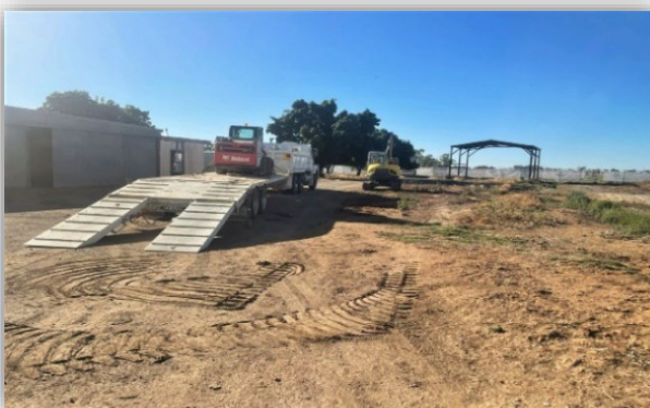
Image 11: VIC1 Stanhope Bioenergy Project site
