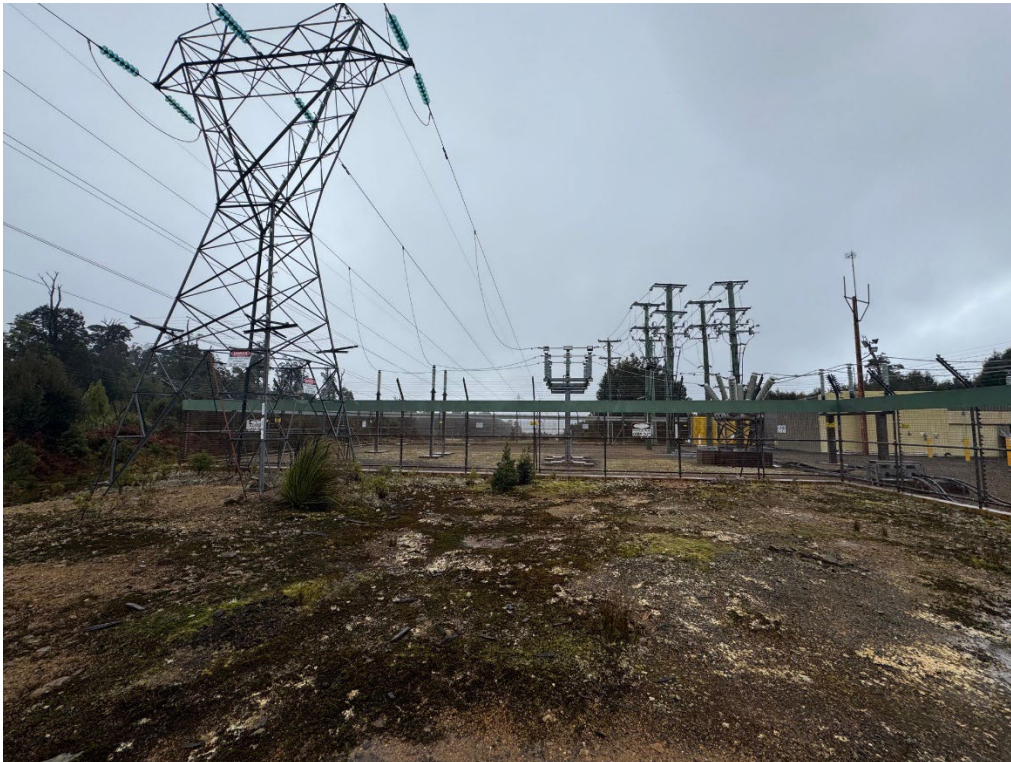
Figure 2 Que River substation; existing power in place
