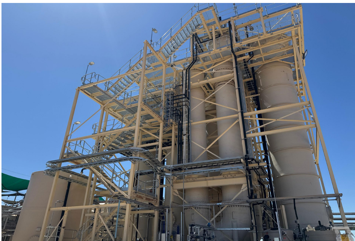
Clean TeQ Water’s CLEAN-IX® U-Column Plant for Heathgate Resources
