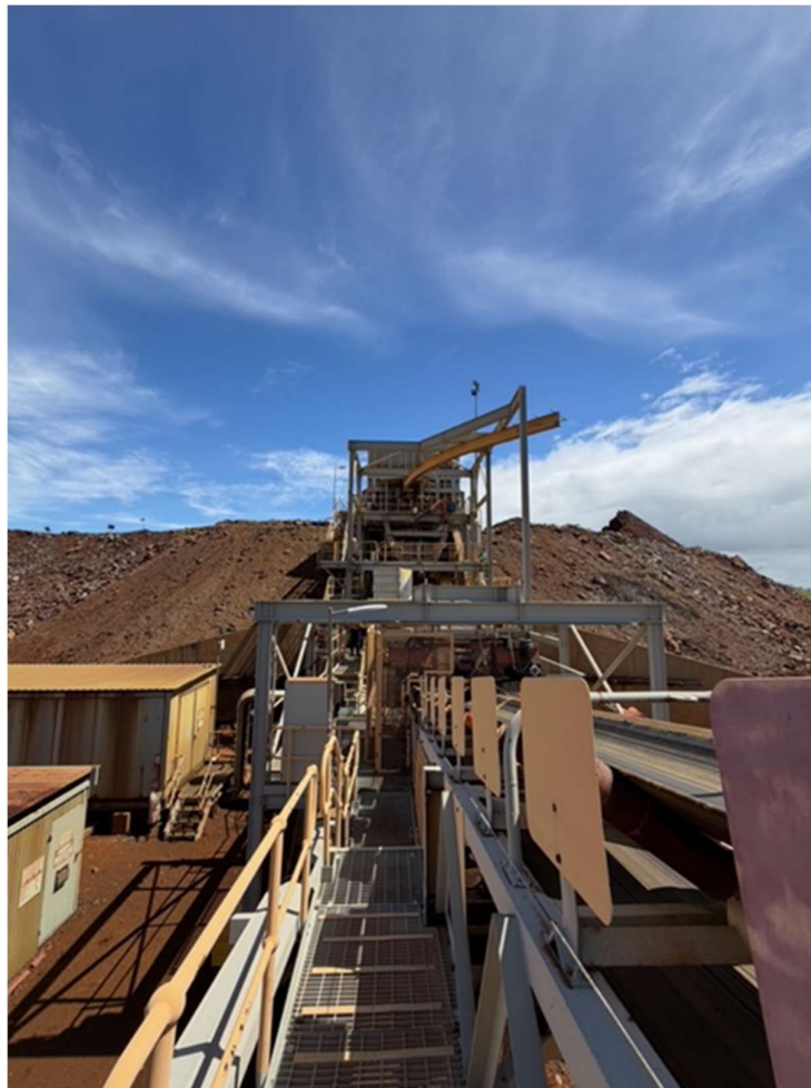
Figure 2: Mill feed Conveyor looking back at Primary Crusher
