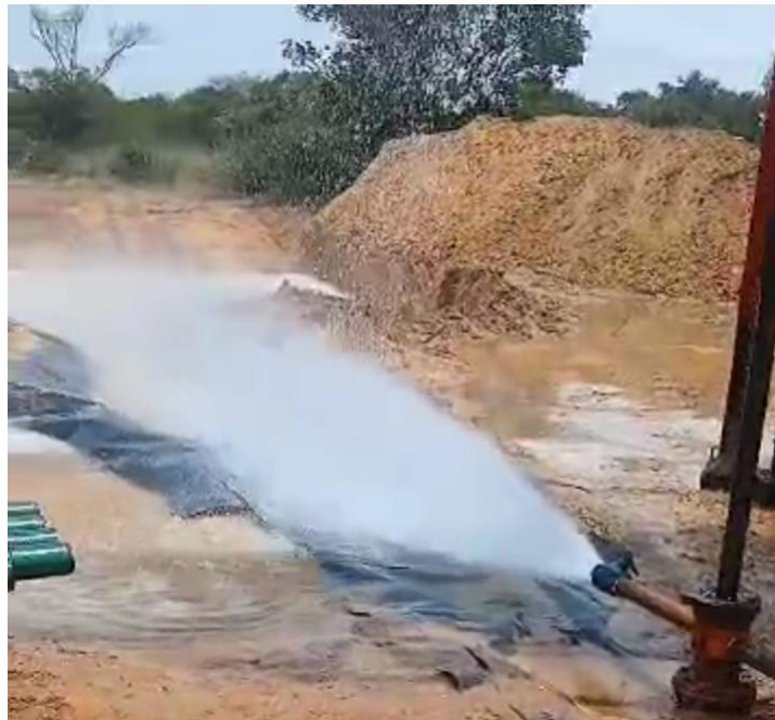
Figure 1. Water flowing from Serowe-3.3 to surface post the initial perforation and jetting water returns. (Source: Botala)
