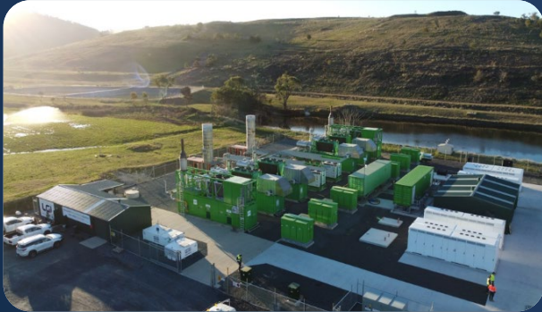
Batteries at Canberra
