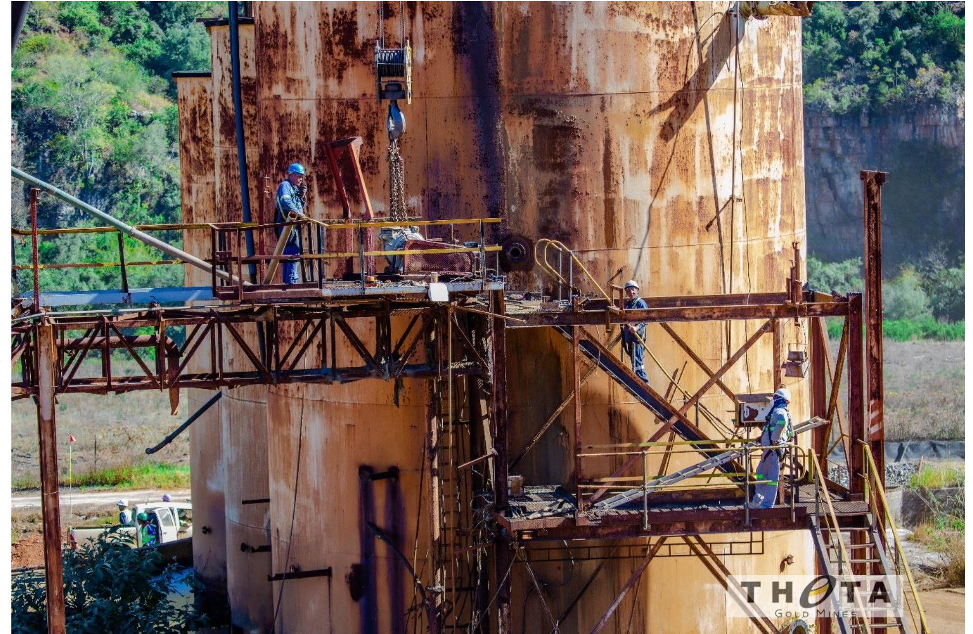
De-commissioning of old plant Leach tanks ahead of site works and construction of new plant
