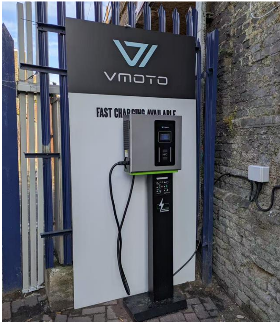
Photo: Vmoto's fast charging station in London, United Kingdom
