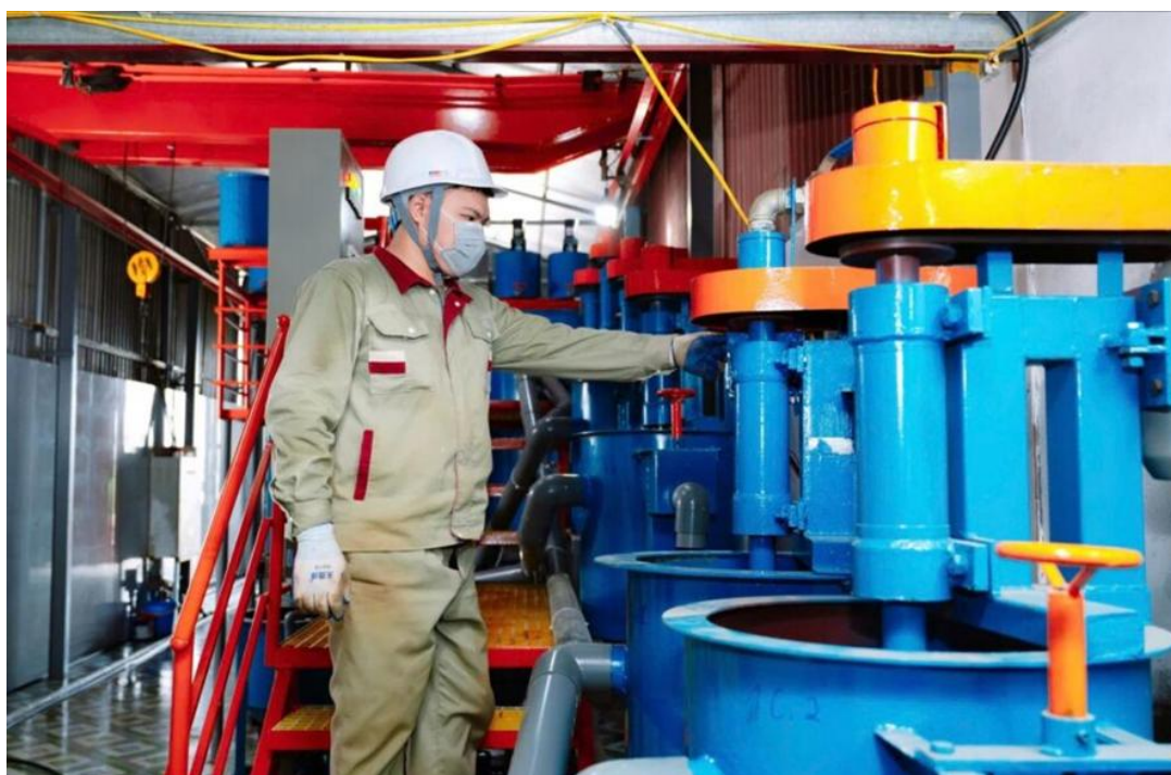
Figure 3: | GAVAQ Pilot Plant – cold commissioning of Pilot Plant
