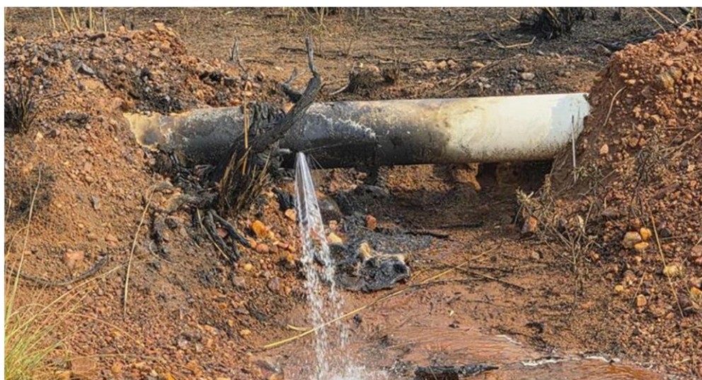
Figure 1: Water pipeline damage due to bushfire
