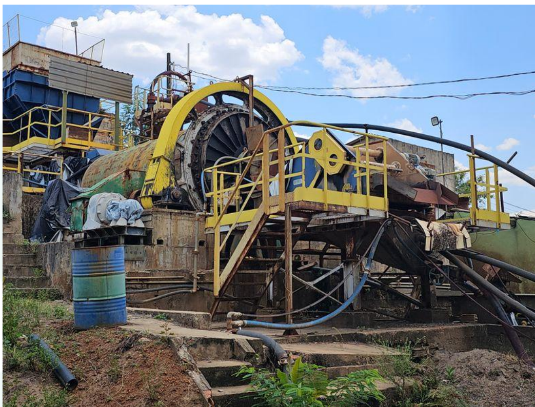
Figure 2: 30tph processing plant (3 rd party owned). 1A
