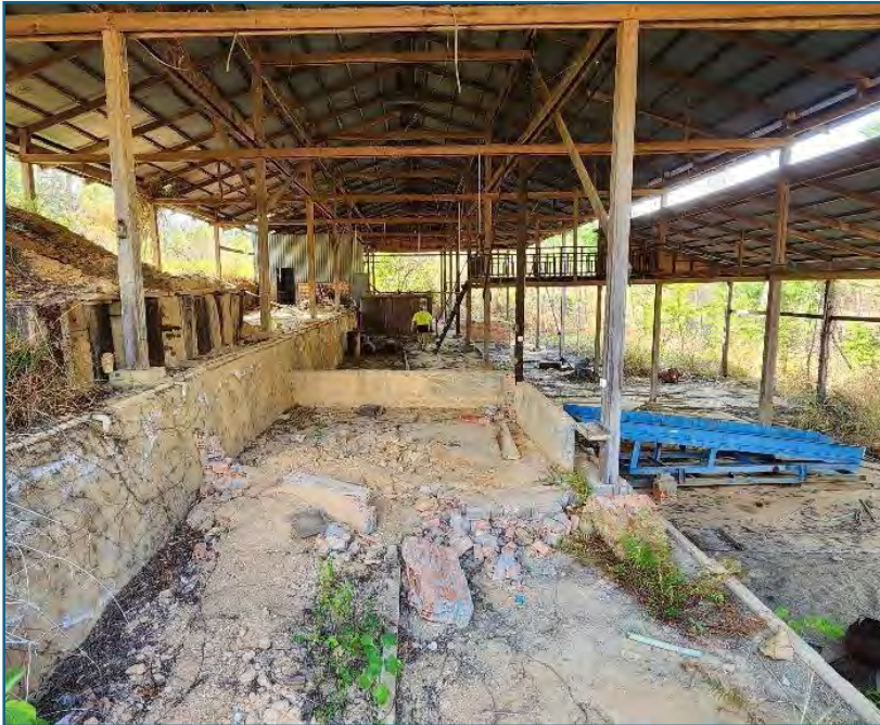
Photograph 17: Gold Metals Group's ore treatment plant in 2024. The plant was closed down in approximately 2020 by the Cambodian Government and now lies in ruin. Source: Author.
