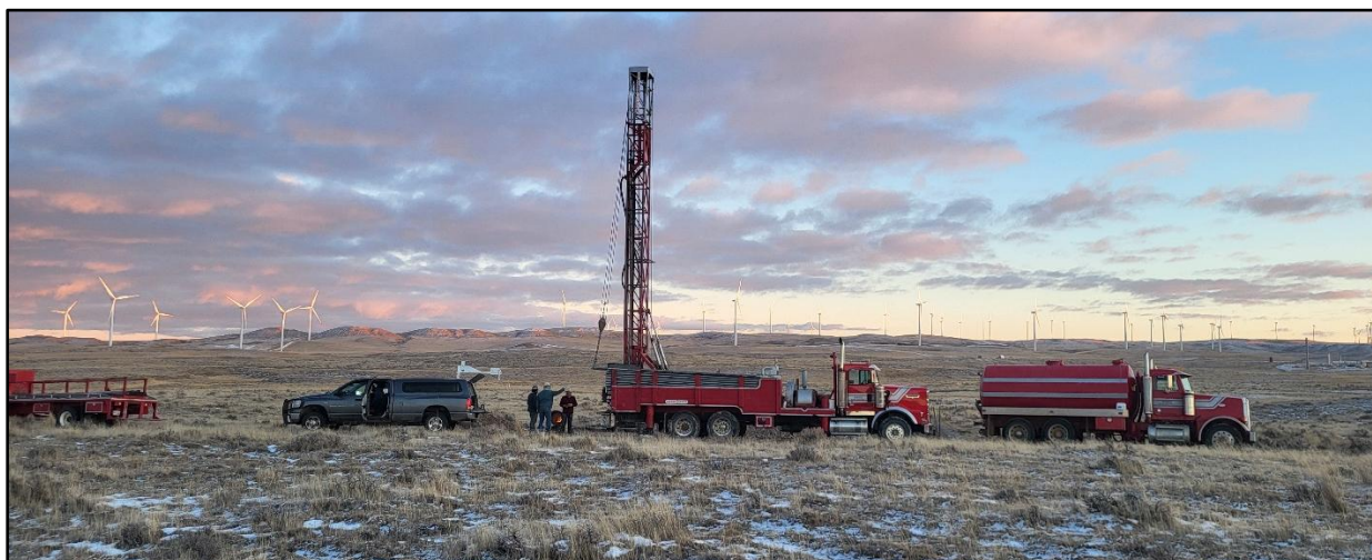
FIGURE 1. MUD ROTARY DRILL RIG AND GEOPHYSICAL PROBE TRUCK NORTH OF MINE UNIT 2
