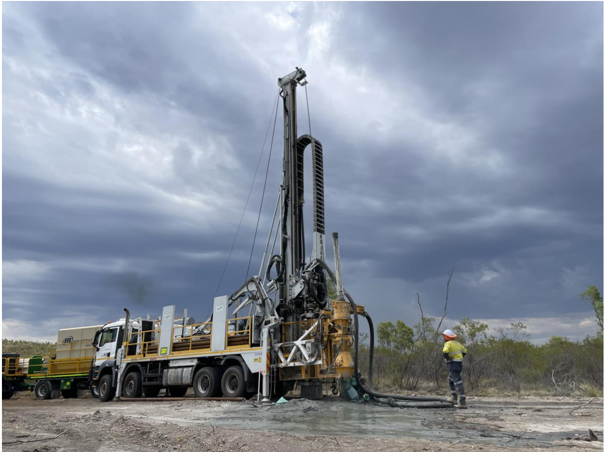
Figure 2: Drill rig set up on first RC drill hole at the Burke Graphite Project (Nov 2025)
