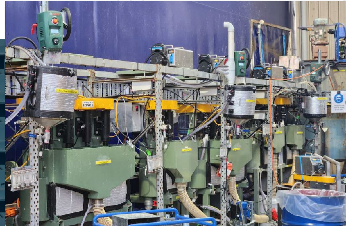
Pilot plant spodumene flotation circuit during operation
