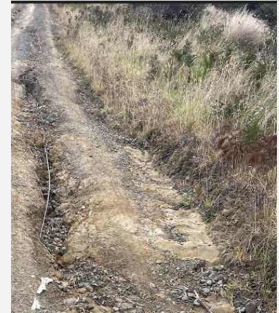
Exposed cable detection
