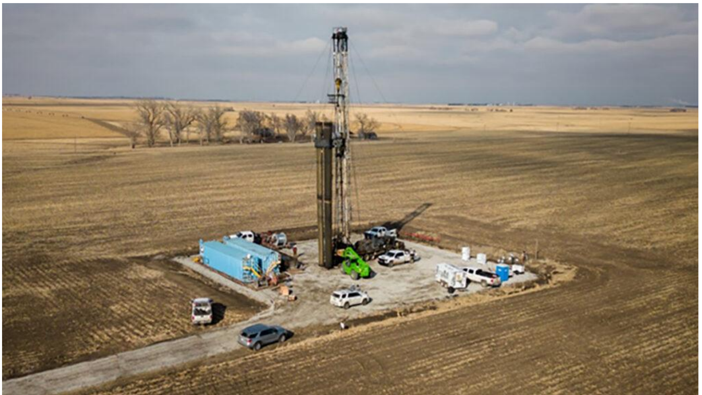
Figure 5. Wildcat well specifically targeting white hydrogen (Hoarty NE3) in Geneva, Nebraska.
