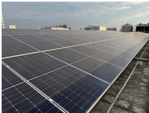
Installation of solar panels on the top floor of the Quanzhou plant 泉州廠區頂樓裝置太陽能板
