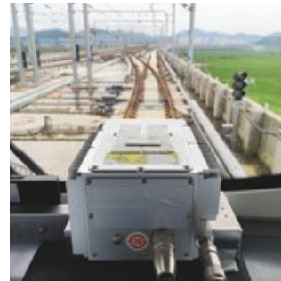
Installed on trains (interior view)
